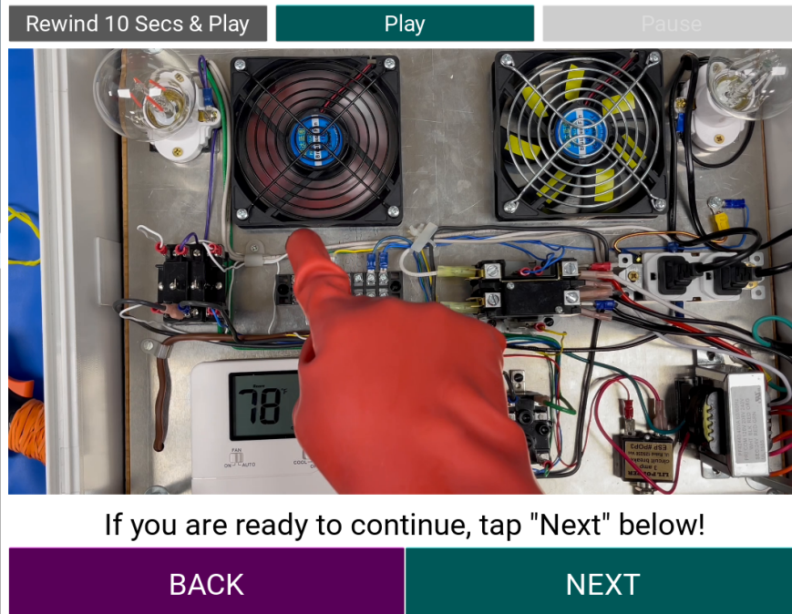
Figure 4.10: Checking Fan's Functionality.
